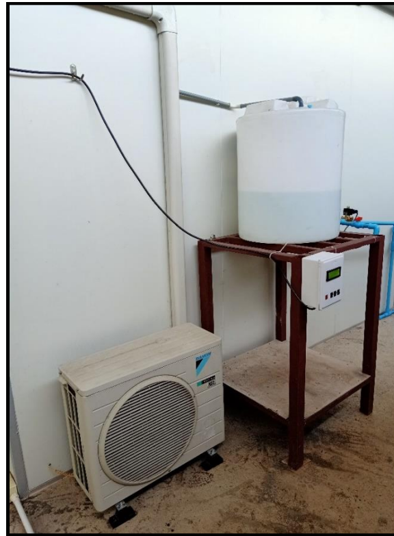
Figure 2: A photograph of indoor room and air conditioning system.
