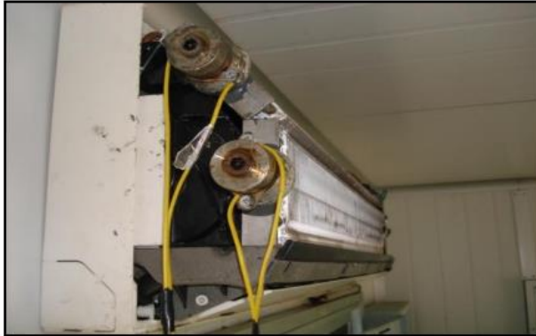
Figure 2 Installation of ultrasonic generators at the evaporator of the tested air conditioner.
